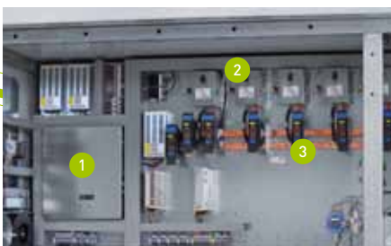
Interior of the CellCube large battery with flow battery controller
